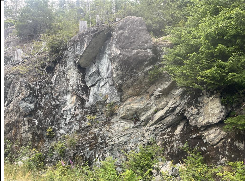
Photo 4: Potential additional rock fall site at 5.2 km.
